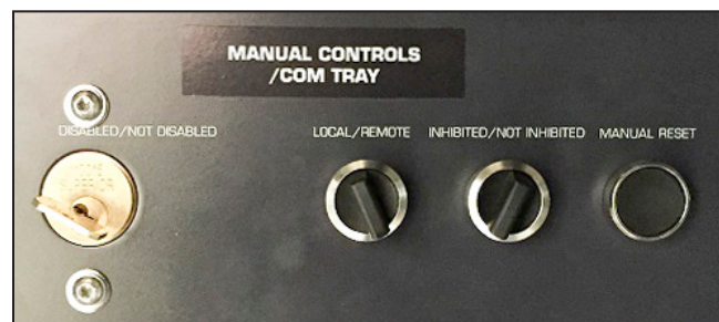
Figure 5. Control panel on the master control rack.
