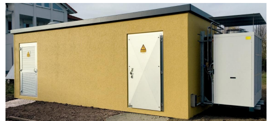
Walk-in STATCOM building with external cooling plant — factory-built and tested before delivery to site
